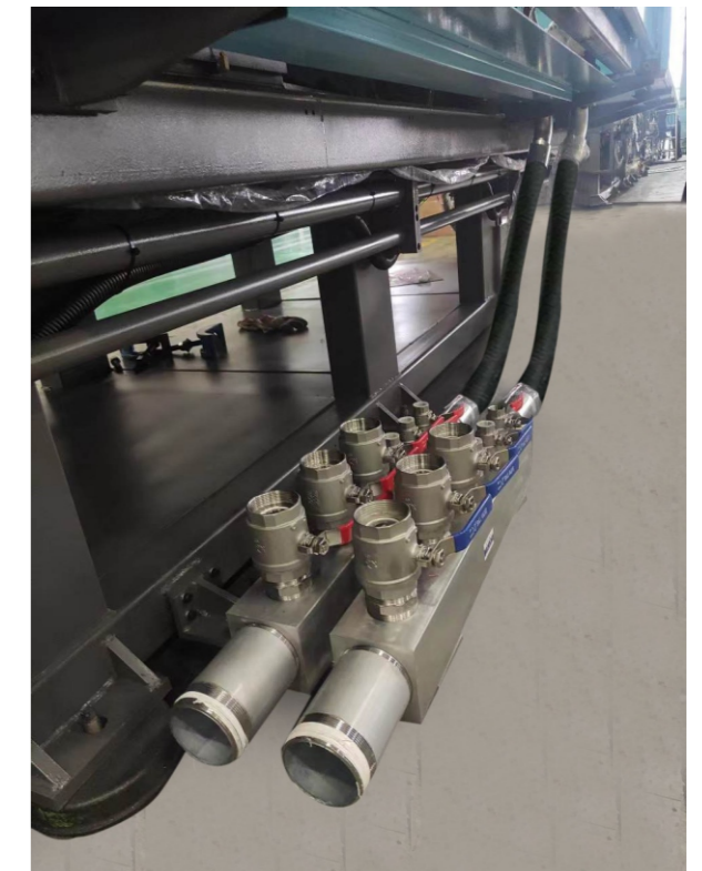
▲ Integrated cooling water circuits
